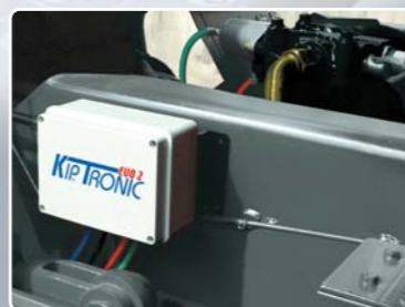
On the CHASSIS: External Box, housing the wiring, the Logic Unit and the pneumatic connections.
